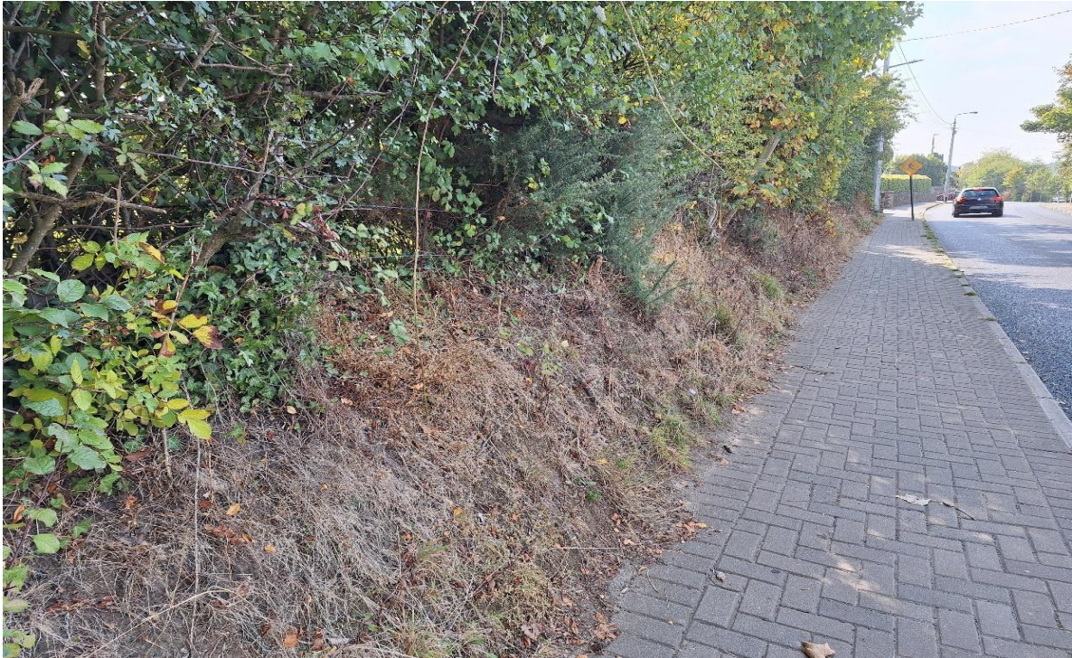
Plate 4-4 Example of a degraded bank possibly due to herbicide treatment
